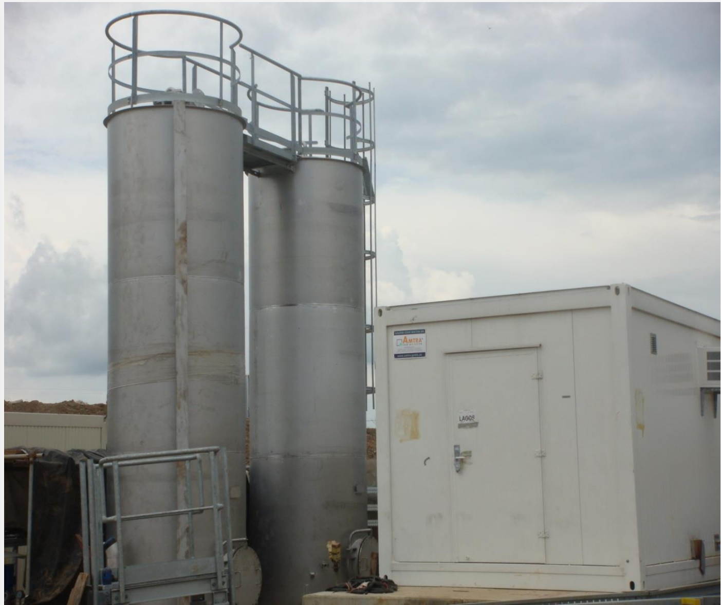
Gas Turbine Power Plant Storage Tank Demineralization Water Tank
