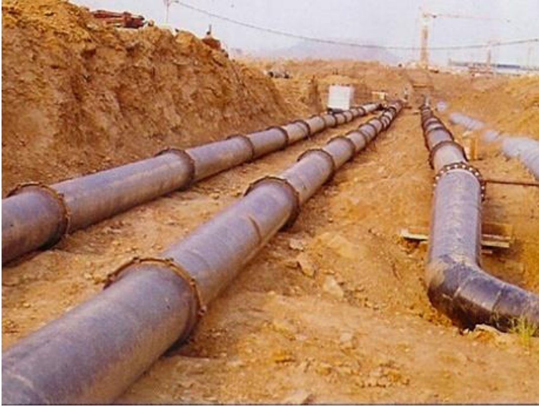
Ajaokuta Steel Plant – Water Supply Lines (3,800 Tons of Cast Iron Pipes)
