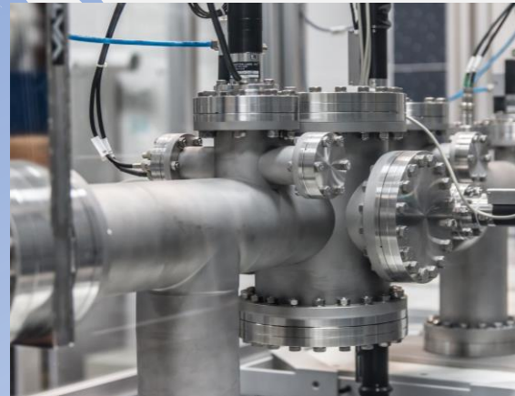
Water Intakes & pumping stations
