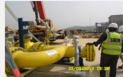
Main Power Plant Gas Receiver, Pressure Reduction/Metering Station.
