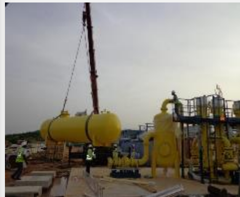
Knock-out Drum & Main Scrubbers for Gas Plant Pressure Reduction/Metering Station.
