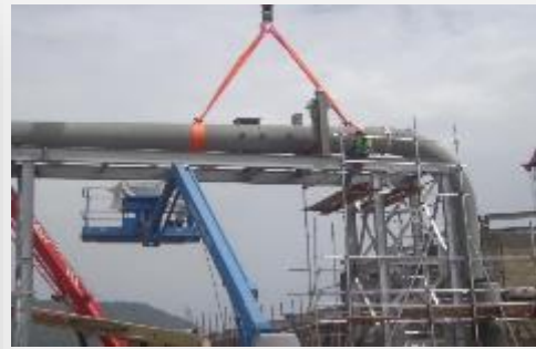
16" Treated Gas Supply Header to individual GT Inlet Gas Scrubbers + Gas PRMS Skids.
