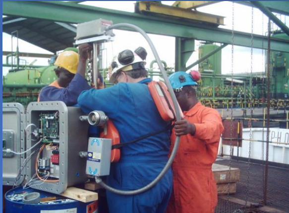
Water cut meter Configuration and Calibration by SDEM
