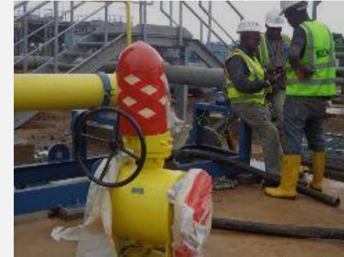
Gas Plant Outlet Piping and Pig Receiver Station.
