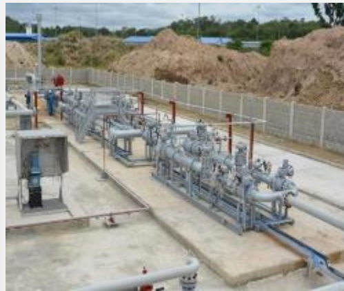
Main Gas PRMS Skid and Interconnecting Piping, Instruments, Control and Power Cabling.
