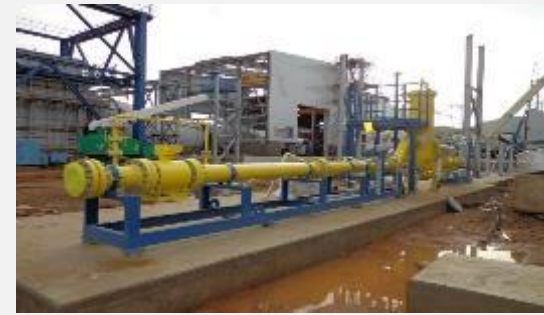
Gas Turbine Inlet Gas Scrubber & Gas PRMS Skid.
