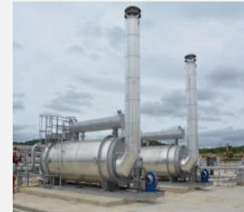
Water Bath Heaters for the Gas Plant.
