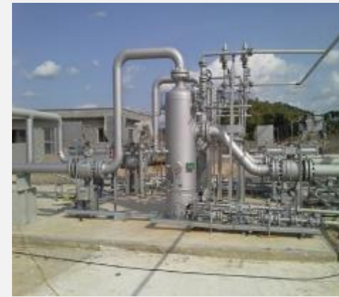
Gas Scrubbers and Interconnecting Piping system network.
