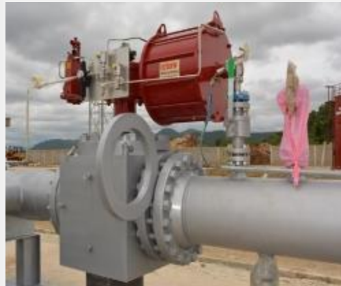
Dual-Operated Gas Line Isolation Valves.
