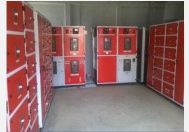
Power & Instruments Control Panels & Equipment
