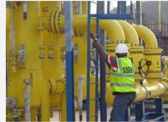
Gas Receiving & Treatment Plant (Commissioned and Hooked-Up).
