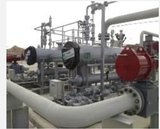
Gas Plant Filter-Separator and associated Piping/Tubing & Instrumentation System.
