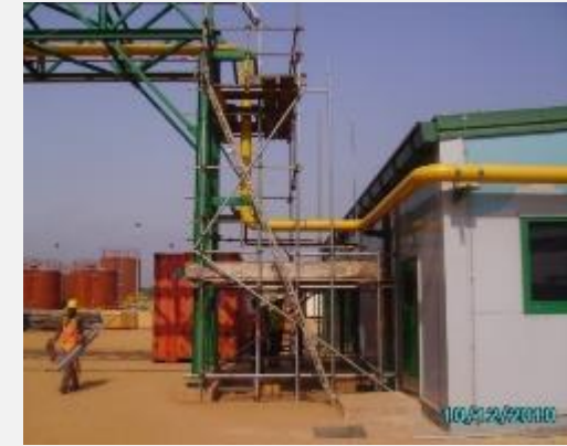
Fuel gas header runs and pipe bridge/support.
